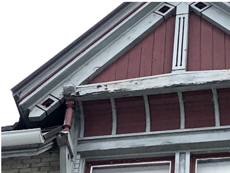
Dramatic before and after of new millwork and paint on third story.
